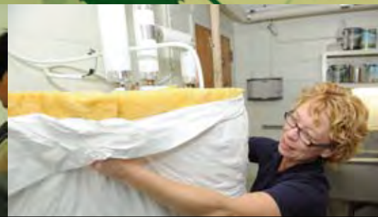
Tammy Wagner, DI Commercial installer, wrapping a hot water tank Photo credit: Dany Abriel
