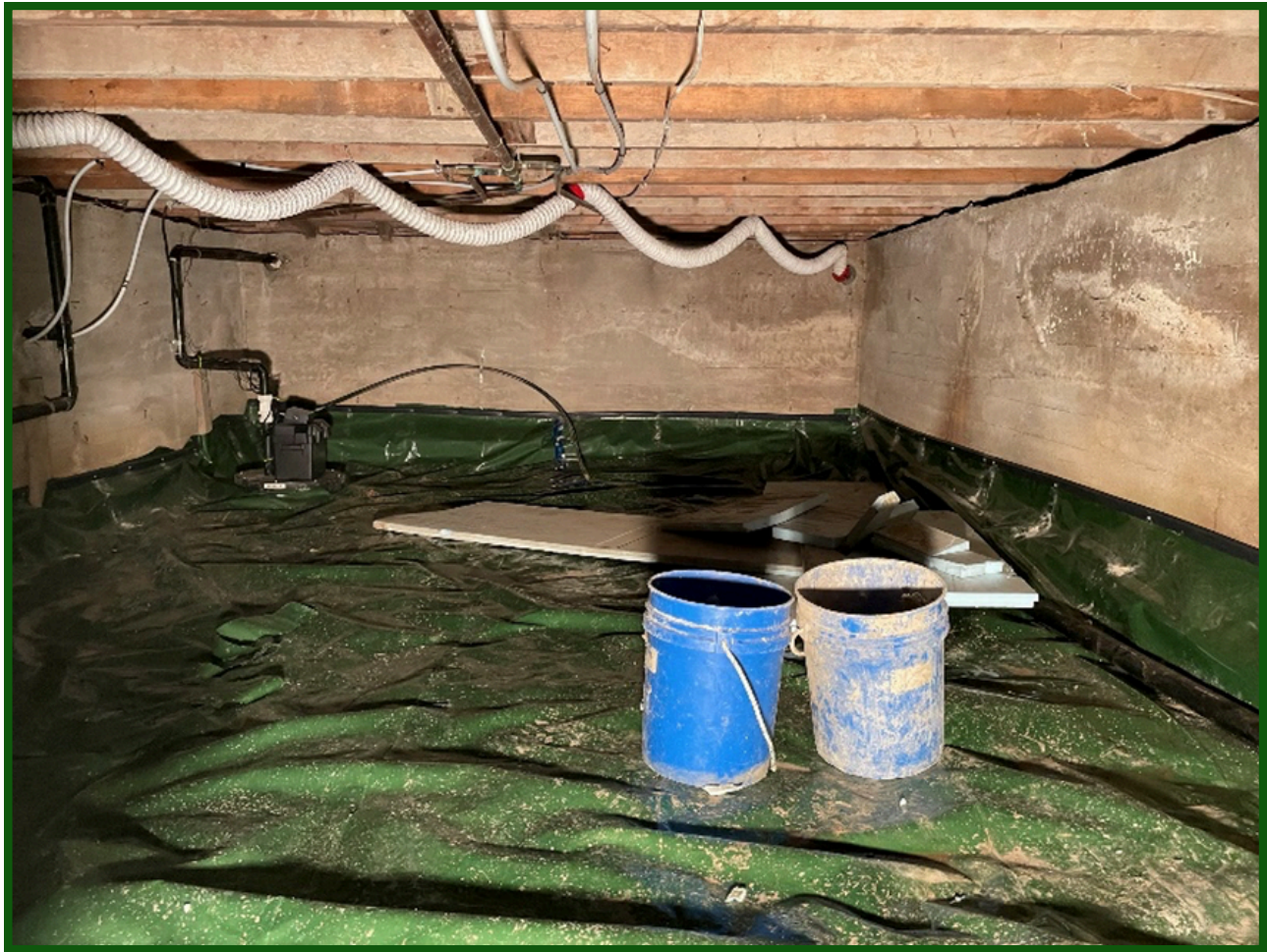
Above: Vapour barrier installed over a crawlspace that has been correctly sealed (Photo courtesy of Clean Foundation ).
