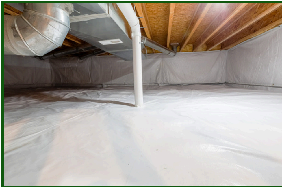
Above: Vapour barrier installed over a crawlspace (Grandbrothers, n.d. via Getty Images/iStockphoto).
