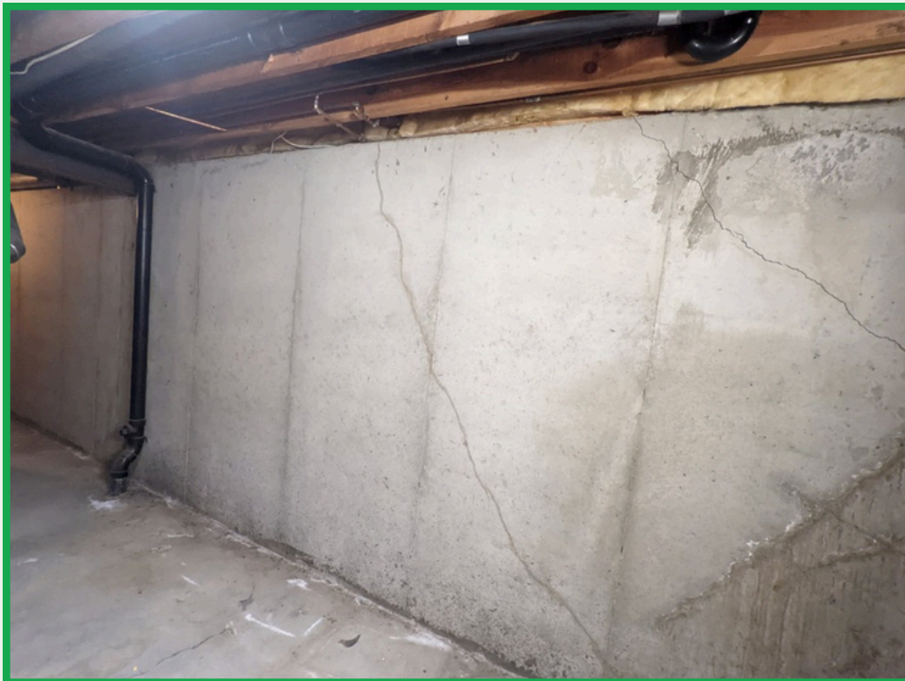
Above: A crack on the interior wall ( Schroeder, 2021 ).
